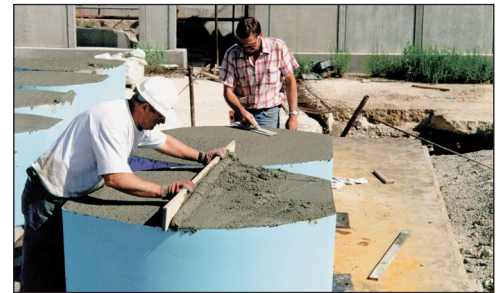
Step 6: Settle and level base of fiberglass shell, allow concrete to cure
