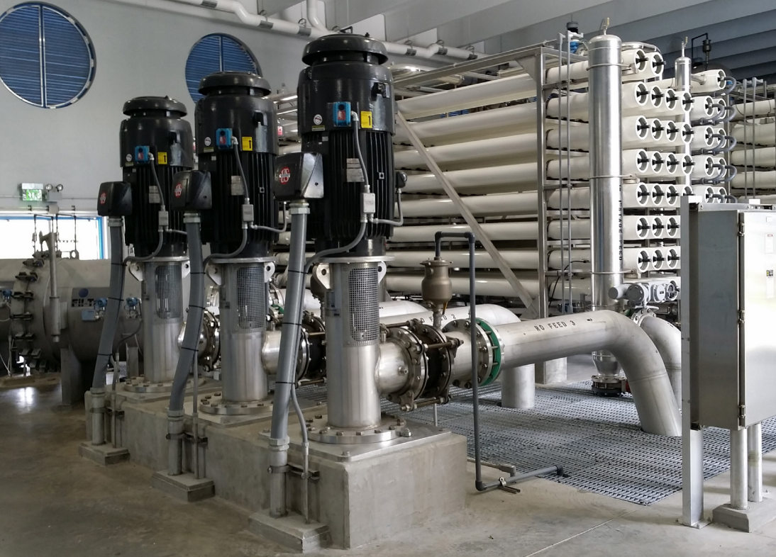
Membrane feed application with Floway Pumps
